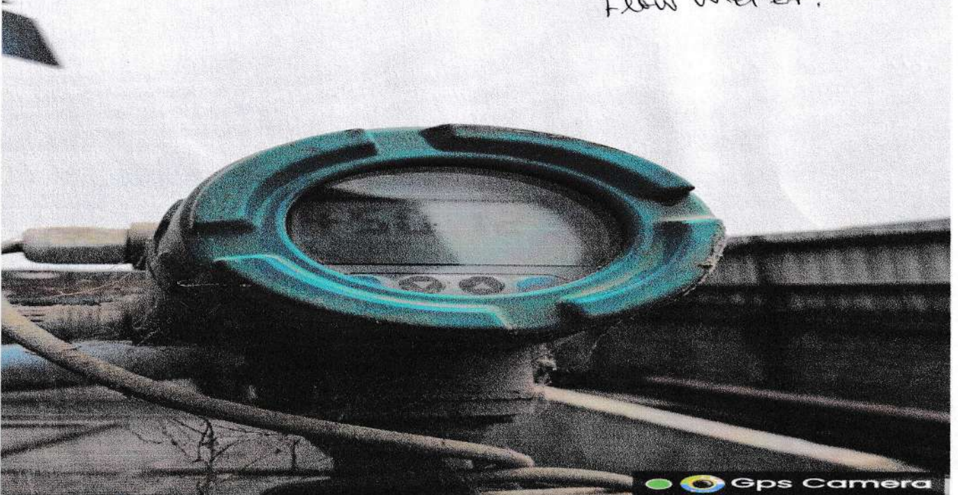
Outlet of ETP Flow meter.
